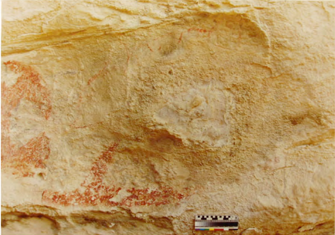
Photo by BJA (1992-3): There are some type of concretions on the surface of the limestone, with an exfoliated-eroded area in the centre. Some flaking can be seen at the bottom and dust towards the top.
