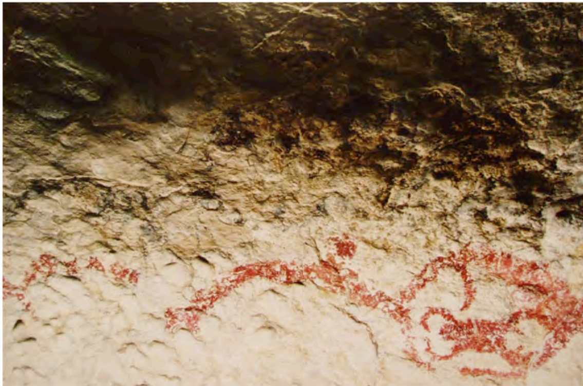
M1' (28.06.2005) : The frame of the photo is larger, so that it is easier to relocate. No further flaking or exfoliation, no change. Surface still black stained.
