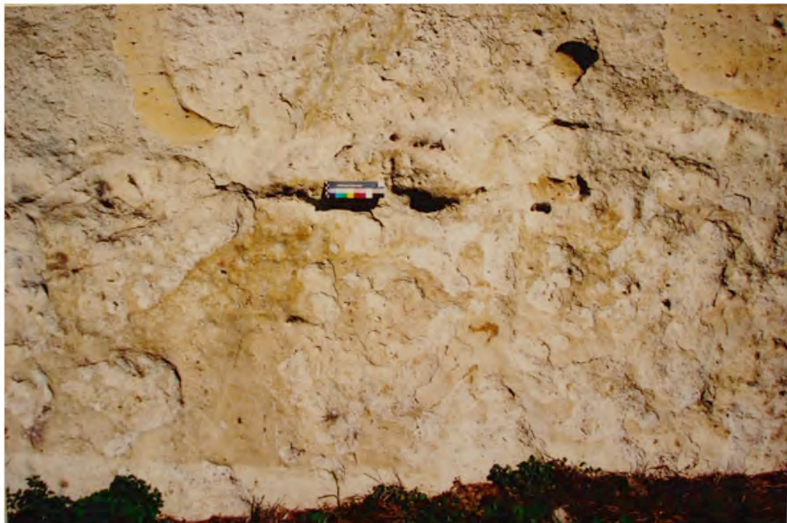
M1 (05.04.2005): Fig 4a, 4b and 4c still visible. No noticeable extension of exfoliation. Bird droppings washed away but new ones have appeared. Vegetation changed in species but not in quantity or volume. There is a dark stain under fig 4b. Surface clearer than before, perhaps due to wetting.
