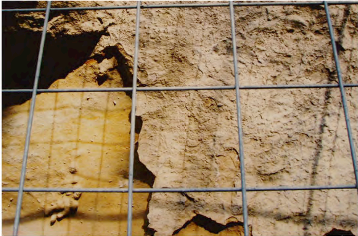
M1" (29.06.05): 2 water flows can be seen in the top of the middle of the photo. There is a lot of dust that shows the direction of the wind and that is exfoliated in several spots. A big piece of rock has been lost, showing salts underneath. The eroded area on the left undercuts the dusty surface. There is some alveolization in the eroded area.
