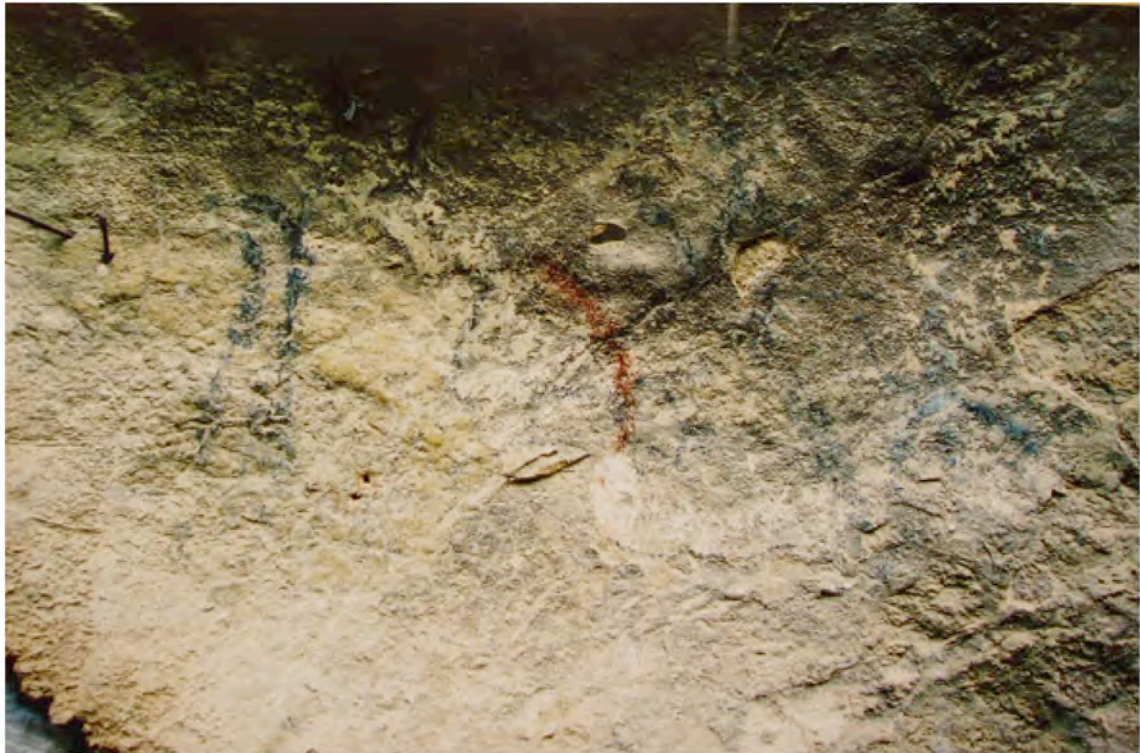
M1' (28.06.2005) : No change to notice. The post has been removed but the nails are still there.
