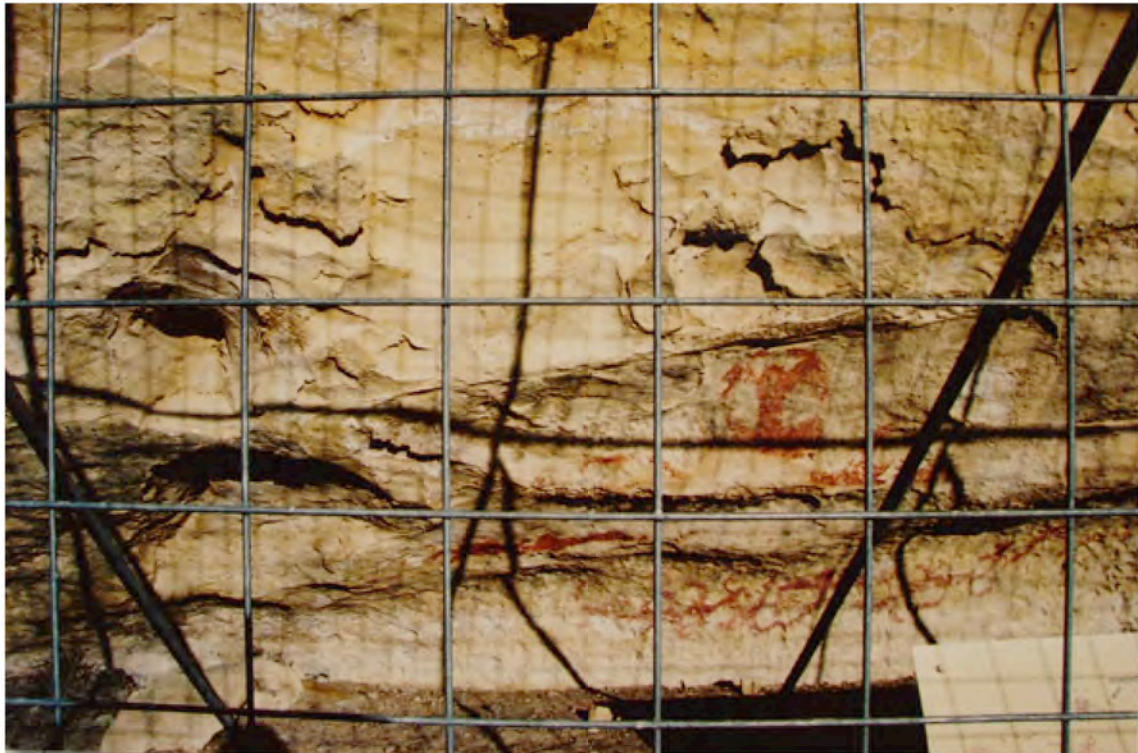
M1" (29.06.05): there are salts forming irregular lines and spots in the eroded area on the top of the photo. There are also salts in a smaller eroded area on the left side of the paintings.
