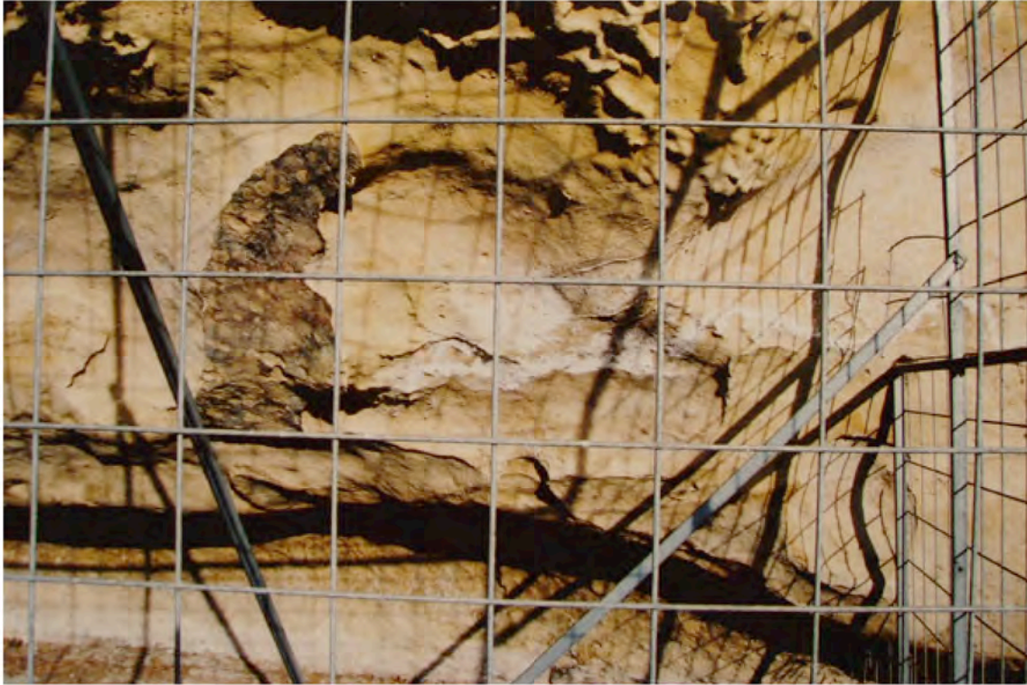
M1" (29.06.05): there are quite a lot of salts, forming lines and crusts on the surface of the eroded area. These are both soluble and insoluble salts (gypsum is not soluble and thenardite is soluble).
