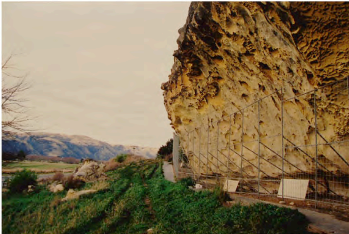
M1' (28.06.2005) : The fence, the road, the boardwalk and the vegetation are the main differences in this photo. All the exfoliated and eroded areas of the cliff face are easy to recognize, so they didn't change too much, their shape is still the same. Even the alveolization is stable. There are many more bushes and trees in the landscape.
