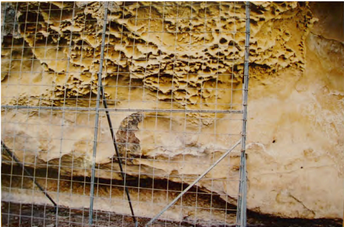
M1' (28.06.2005) : Fig 92 is still visible. The ground has less dung. The alveolization is still there but coarser: some areas of previous alveolizations have become areas of erosion. Salts can clearly be seen forming a line from fig 92 towards the alcôve, and there are many more salts in the alcôve. The darker area caused by stock rubbing is less visible, and it seems that there is moss or algae growing in the alcôve.
